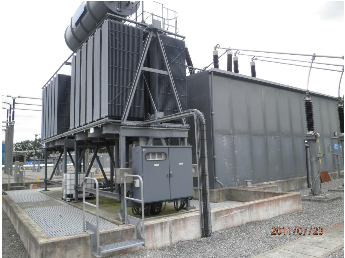
Plate 4.9 Typical (large 400kV) power transformer
